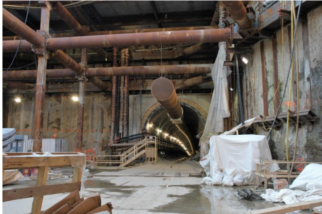
Strut-and-post bracing of cutter soil mix walls for the North Shore Connector Project
