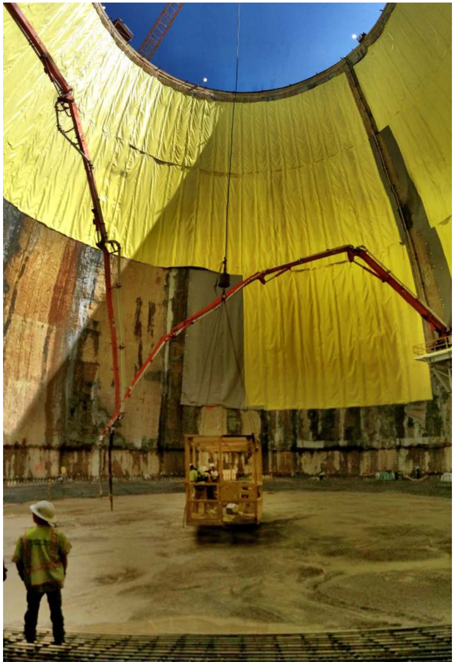
JCK Underground staff provide program management services for DC Clean Rivers Project.
